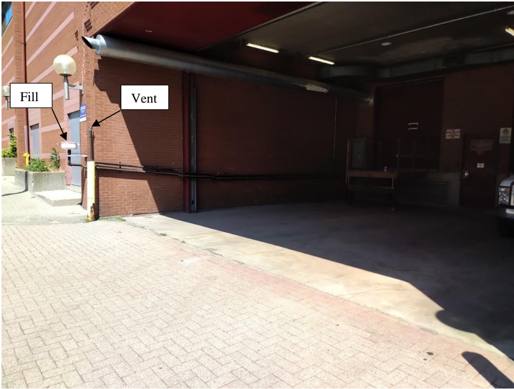
Photograph No. 11 – Northwest facing view of a potential fill and vent pipe (PCA 28) located at 1 Market Street from Colborne Street East.
